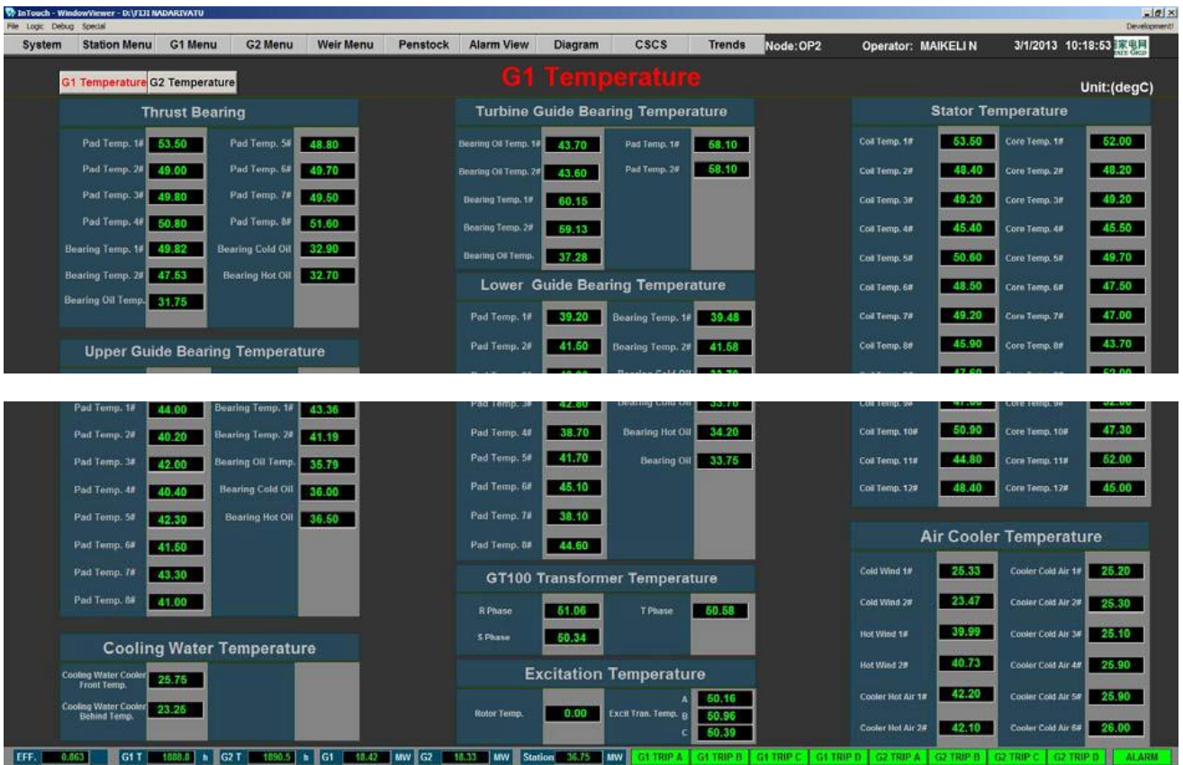
Figure 9-14: Generator Temperature Monitoring Screen
