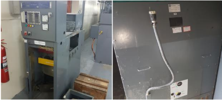
Figure 9 : Old switch gear room scrap 4
