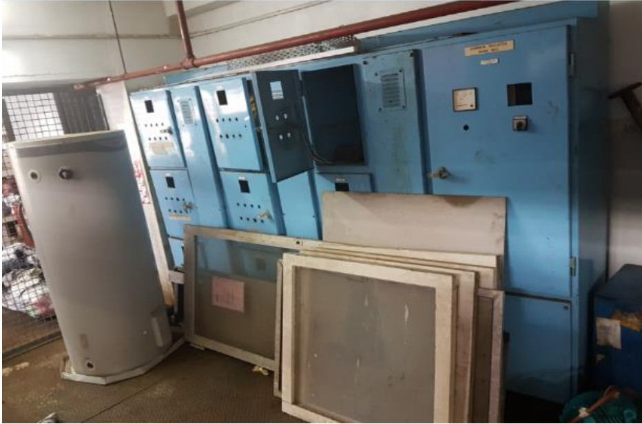
Figure 11: Motor control center panel
