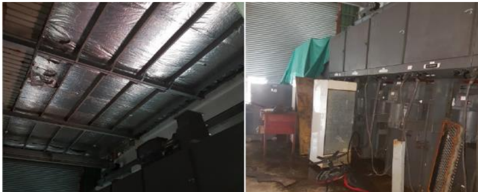
Figure 8 : Old switch gear room scrap 3
