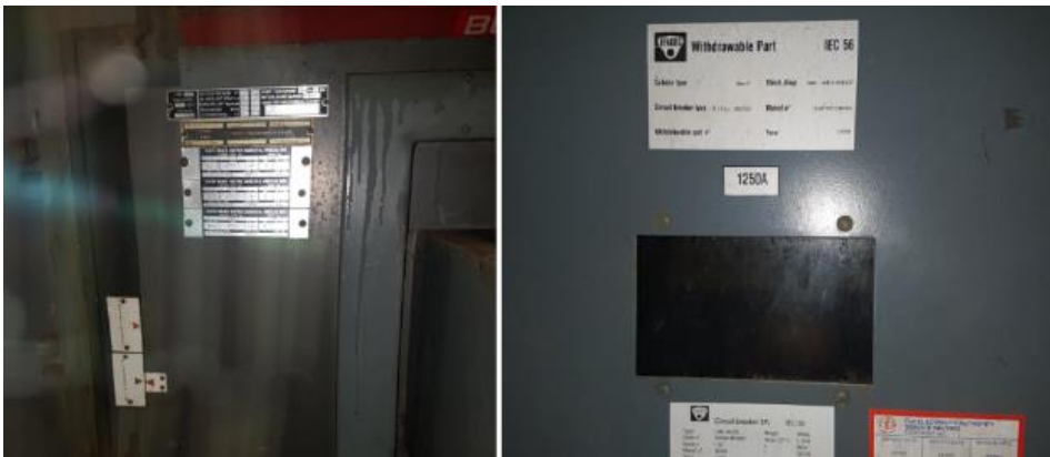
Figure 10 : Old switch gear room scrap 5
