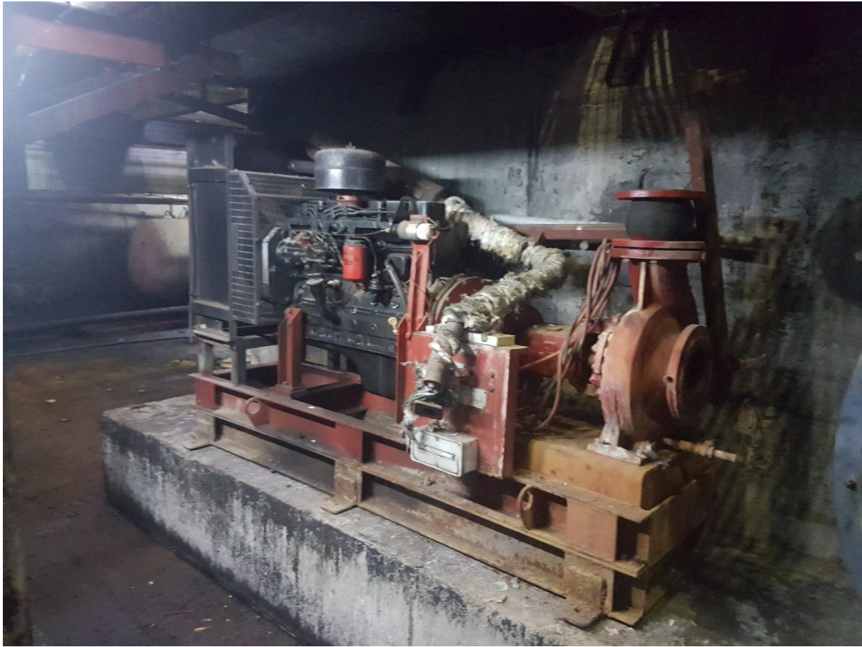
Figure 1 Old Kinoya Fire Pump
