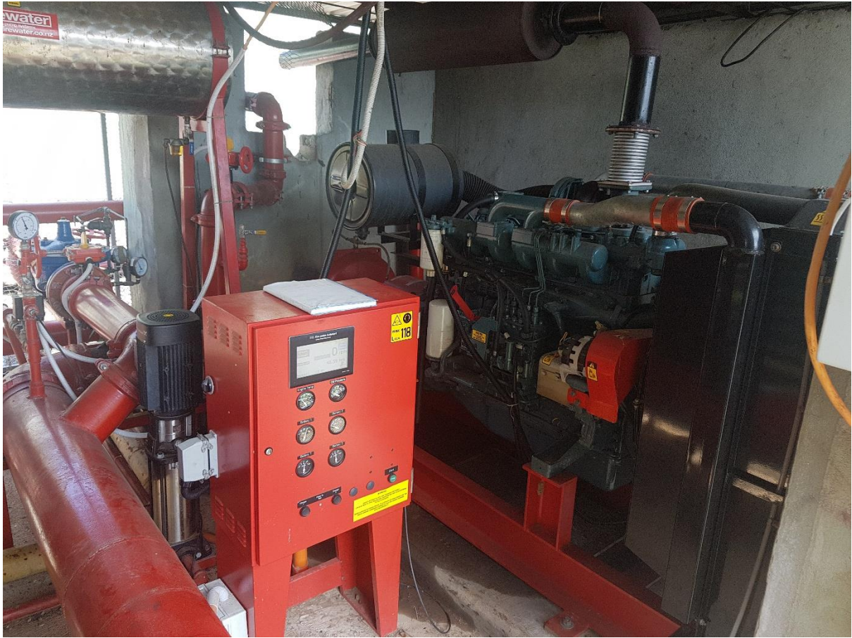
Figure 2 New Kinoya Fire Pump Unit
