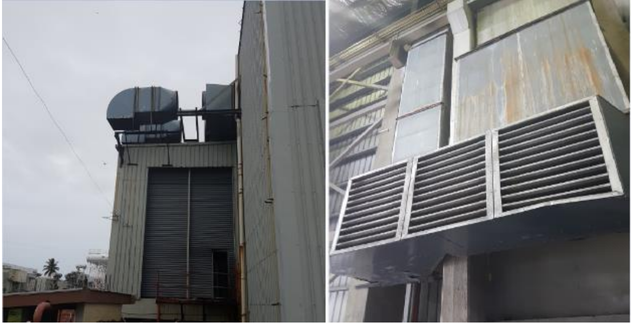
Figure 7 : Old 33kV switch gear room scrap 2
