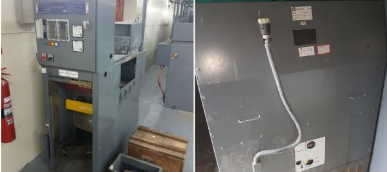
Figure 9 : Old switch gear room scrap 4
