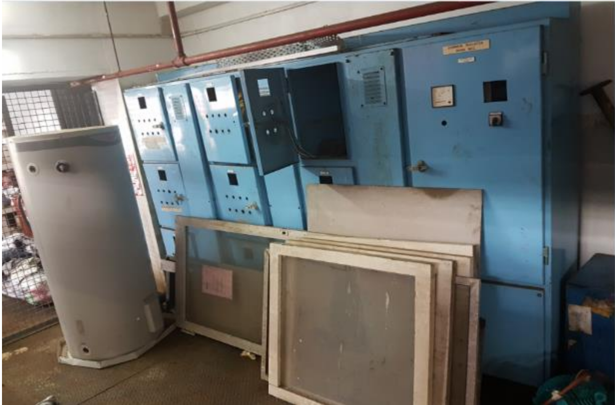
Figure 11: Motor control center panel
