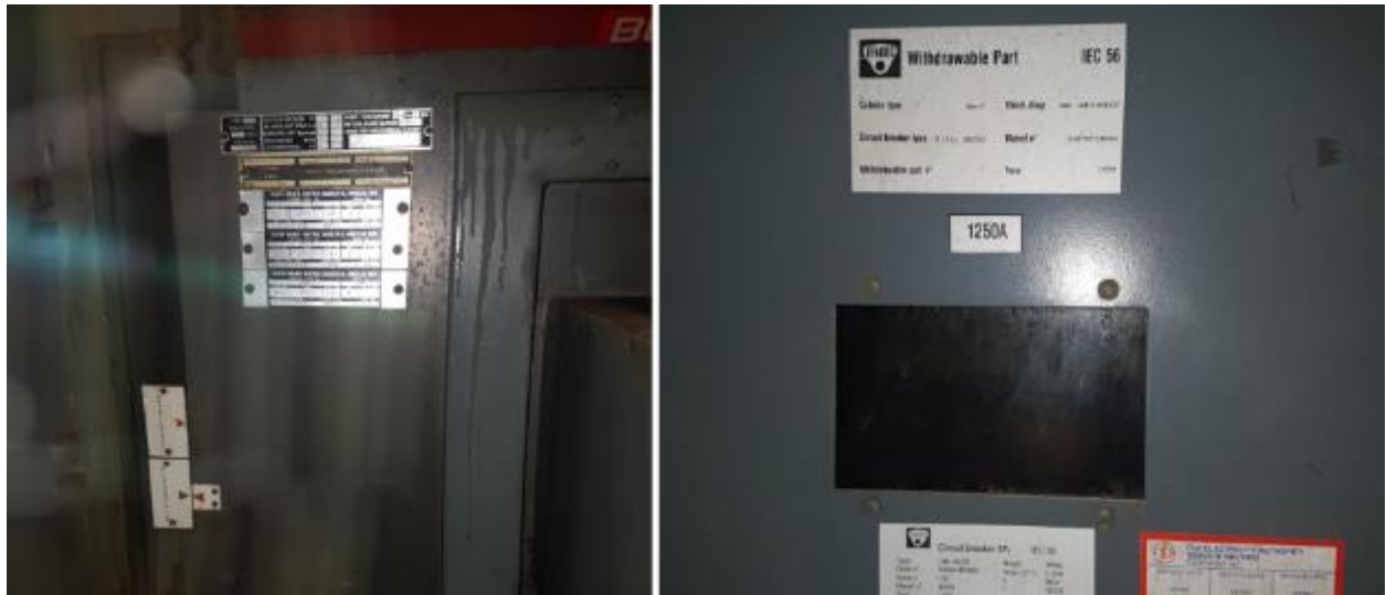
Figure 10 : Old switch gear room scrap 5
