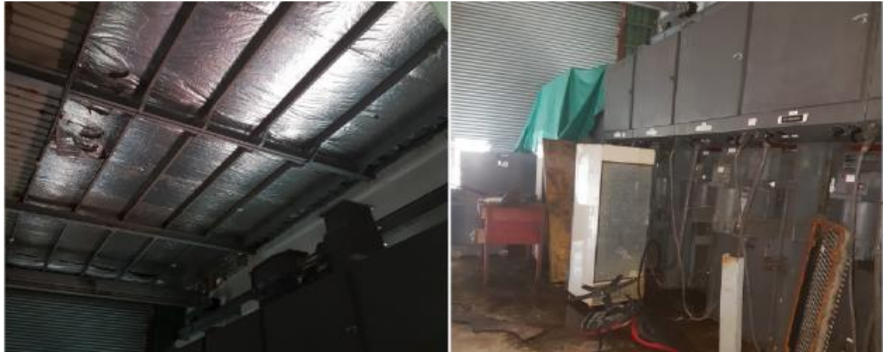
Figure 8 : Old switch gear room scrap 3
