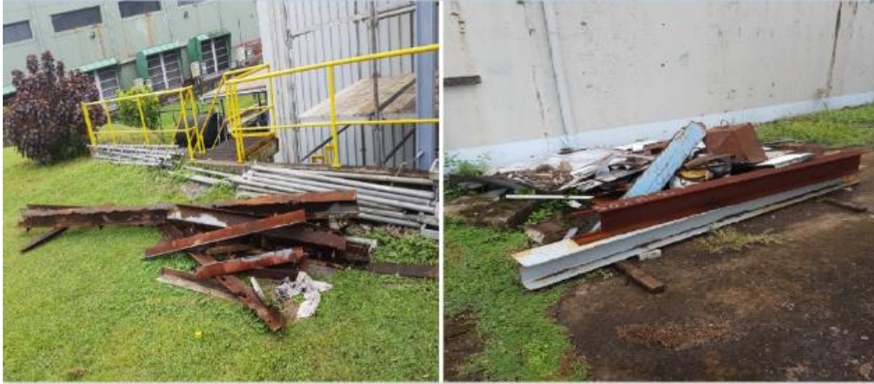
Figure 13: Scrap at the back of Power Station
