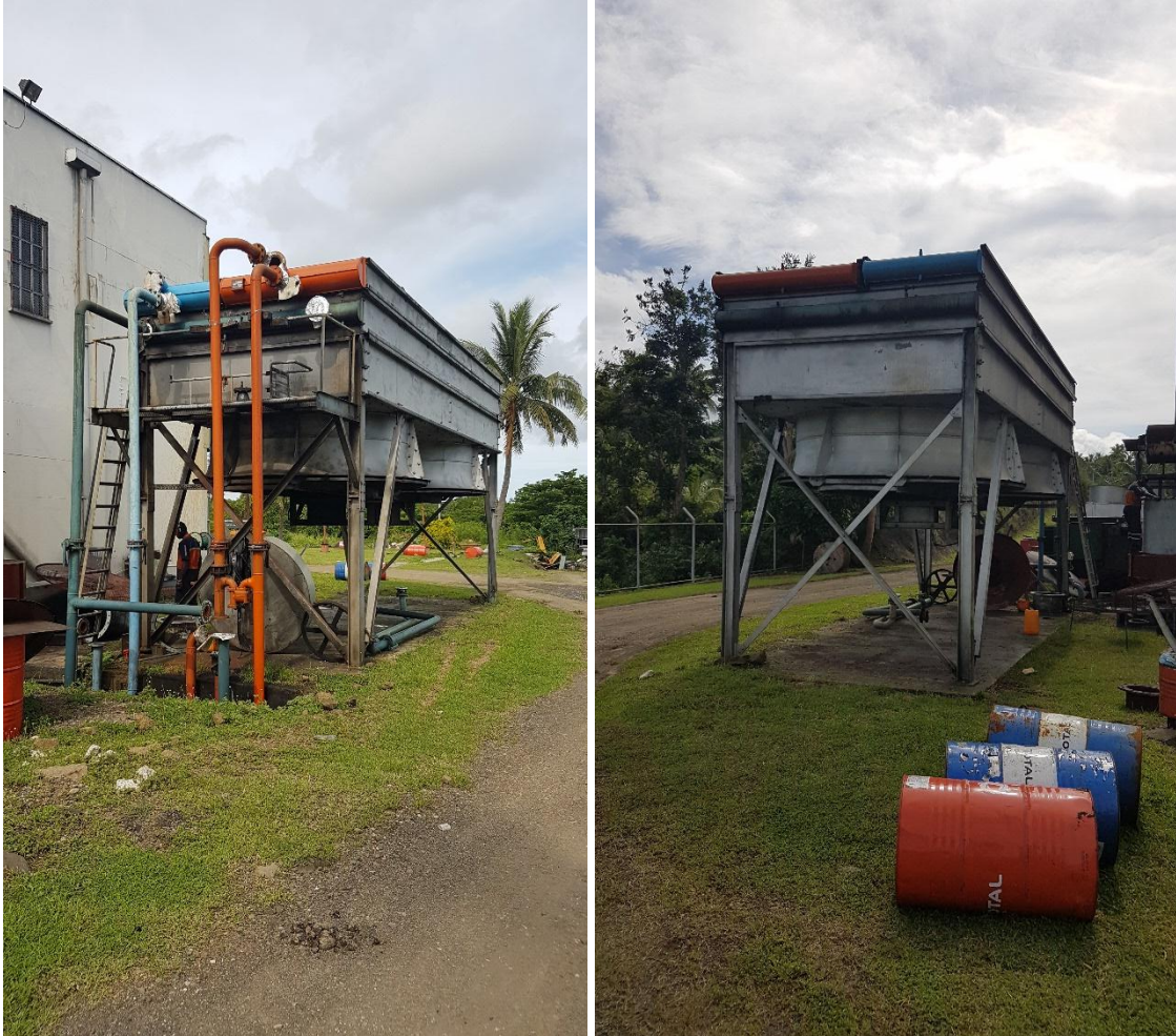
Figure 2 Photo of G6 Current Radiator Setup
