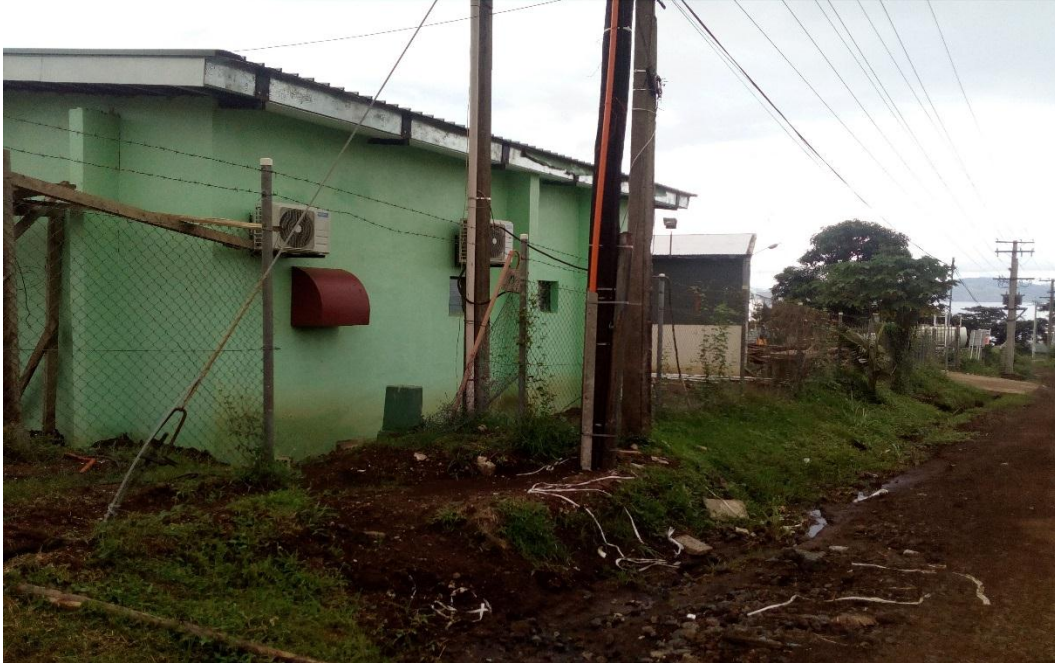
Fig1. Section of fence where chain link is missing
