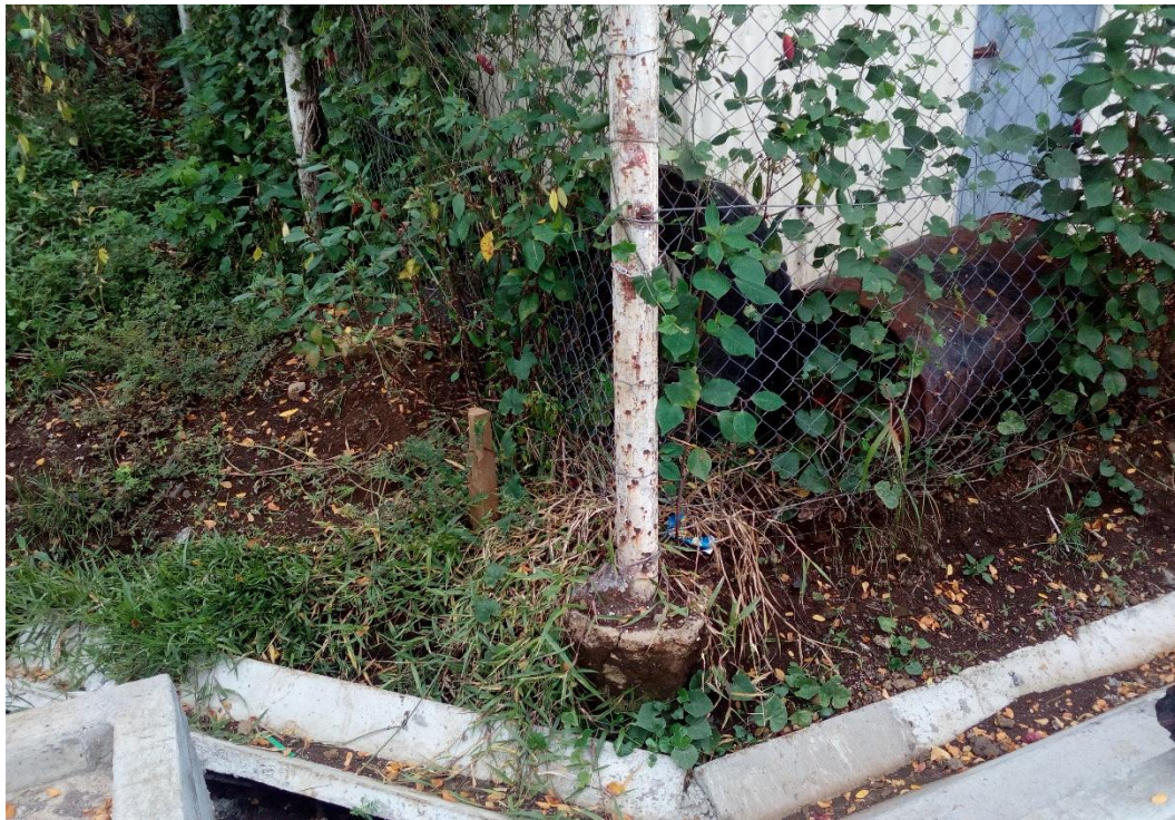
Fig 2. Supporting poles showing rust and concrete setting exposed
