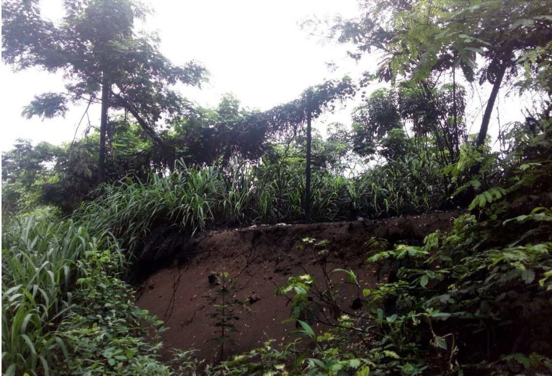
Fig 3. Poor support for poles due to washed away land
