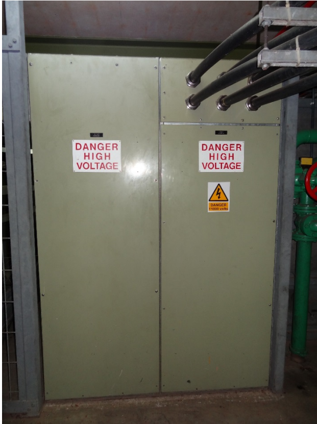
Figure 3 - Rear View - Cables from Generator
