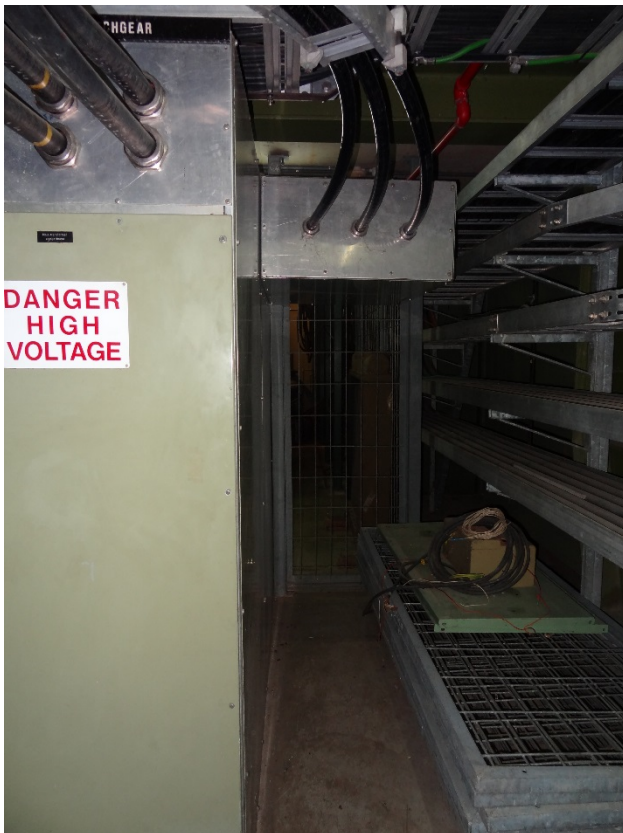
Figure 2 - Front View - Cables to Auxiliary Transformer (Units 1 and 2 only)
