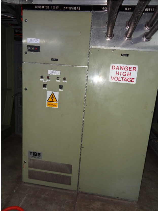
Figure 1 - Front View - Cables to Unit Transformer
