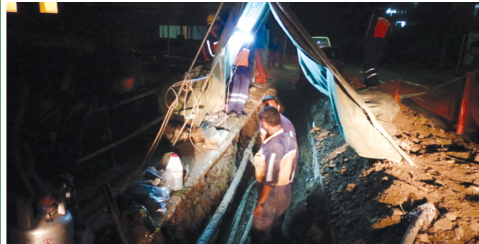
FEA employees carrying out work on underground cables at the Rokobili Power Station in Suva as part of the Contingency Plan to install 40MW of containerized diesel gensets to supplement the low power generation output from Monasavu and Nadarivatu Hydro Schemes due to low rainfall received during the year.
