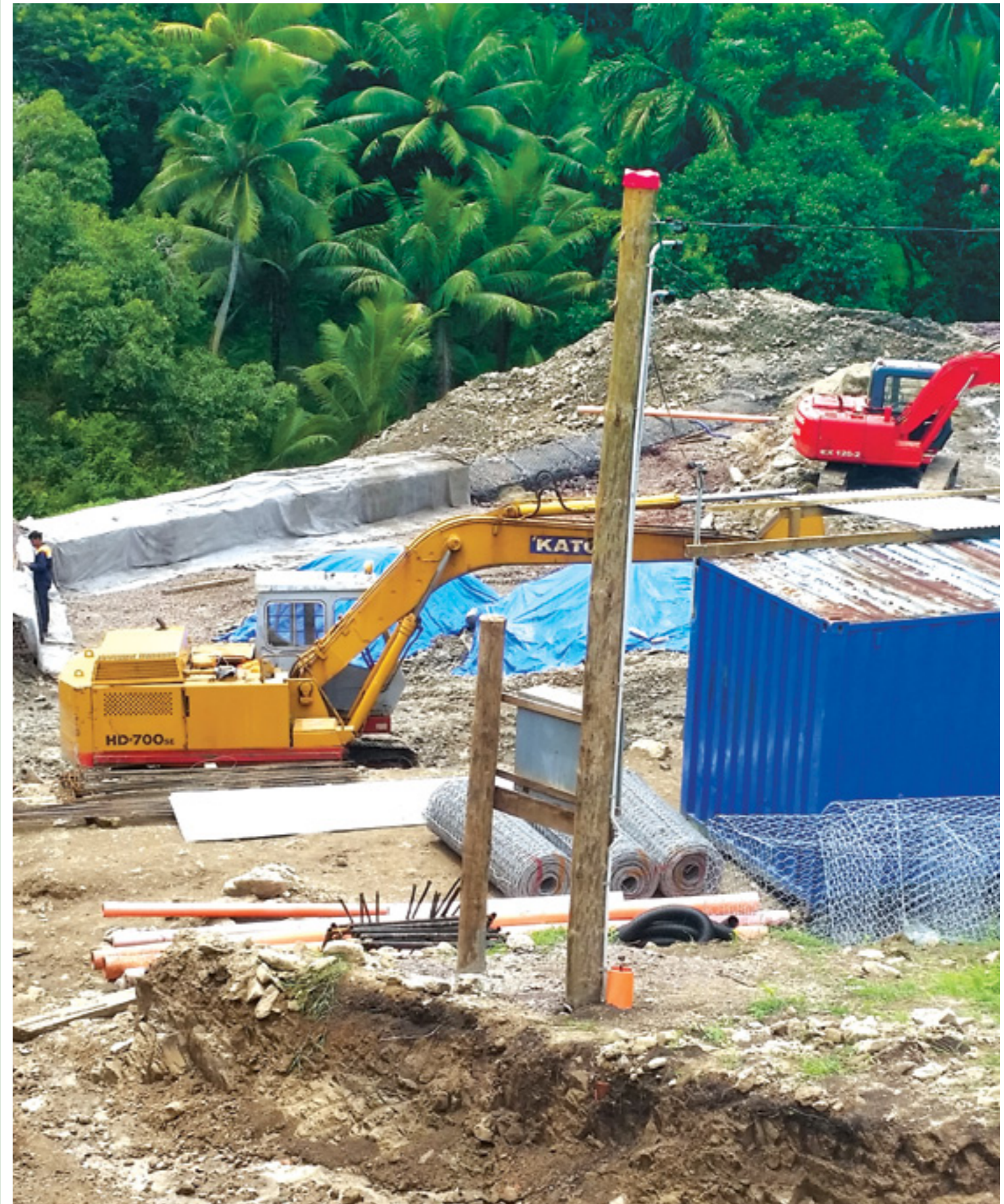
FEA acquired the land for the zone substation off Knolly Street, Suva and commenced construction of the new 33kV/11kV Substation. The total cost of this project is around $17M.
