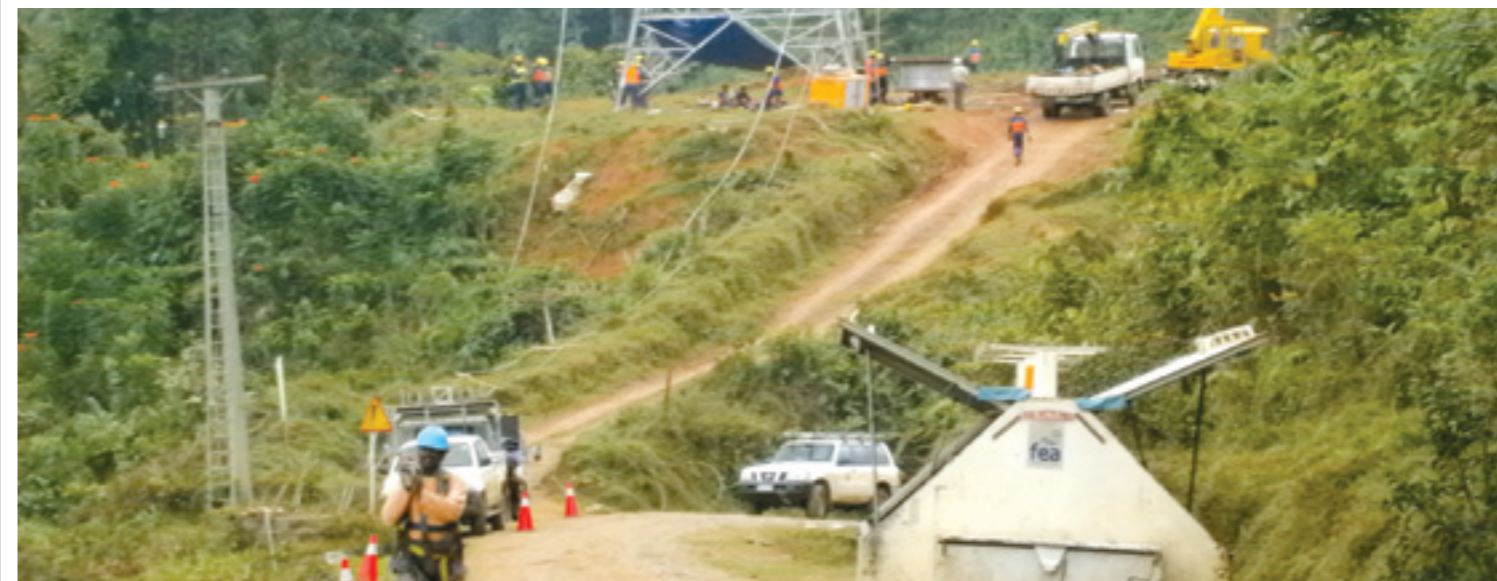
The picture shows work in progress to relocate two steel towers. FEA successfully completed the work to relocate Tower 9 and Tower 98 on the 132kV Wailoa - Cunningham Road transmission line.
