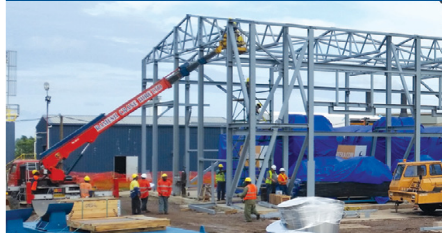
Work in Progress on the installation of the 35MW HFO Generator sets at the Kinoya Power Station. The Project is estimated to cost around $73M and will be completed in late 2015.
