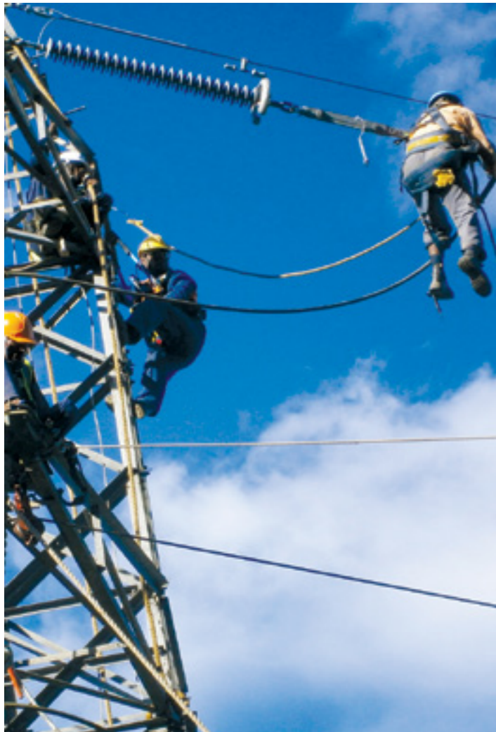
Because of the inherent danger in dealing with electricity, extensive education and training is essential to ensure the safety of FEA workers.
