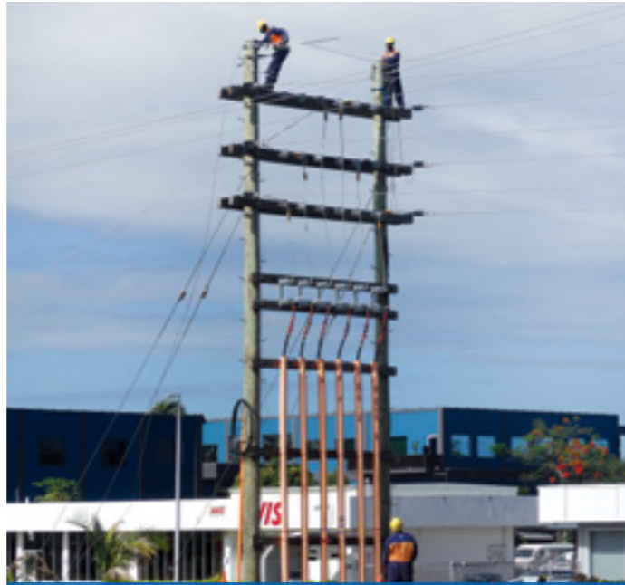
The newly constructed 33,000volts double circuit transmission line from Vuda to Waqadra to improve the security of power supply to Nadi, Sigatoka and Korolevu areas.
