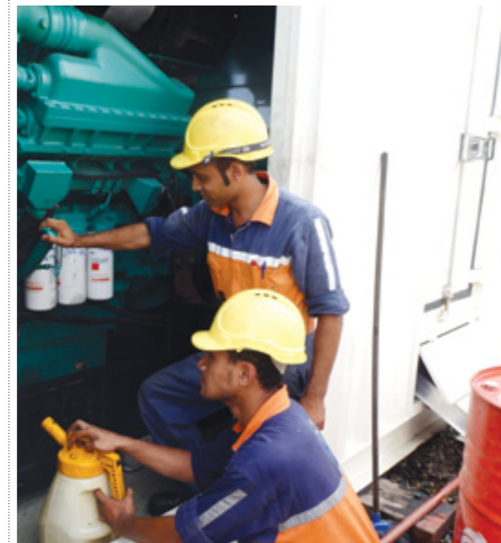
FEA personnel carrying out maintenance works on one of the diesel generators at Rokobili Power Station in Suva.
