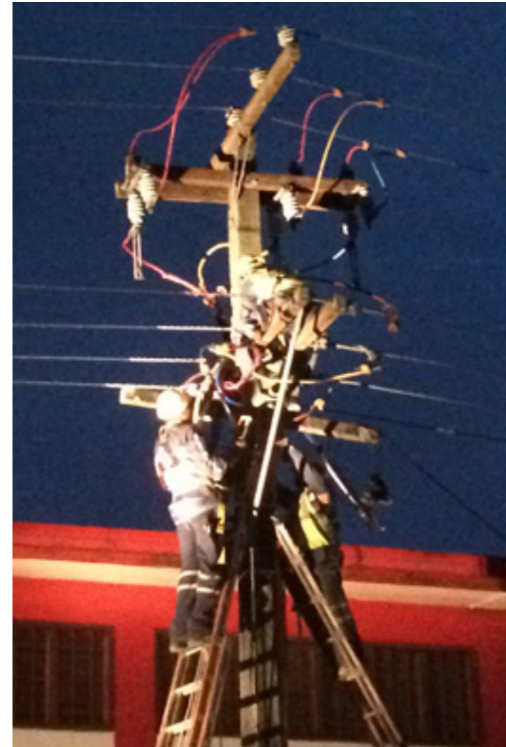
FEA personnel carrying out repairs to damaged power lines at night to restore power supply to customers.
