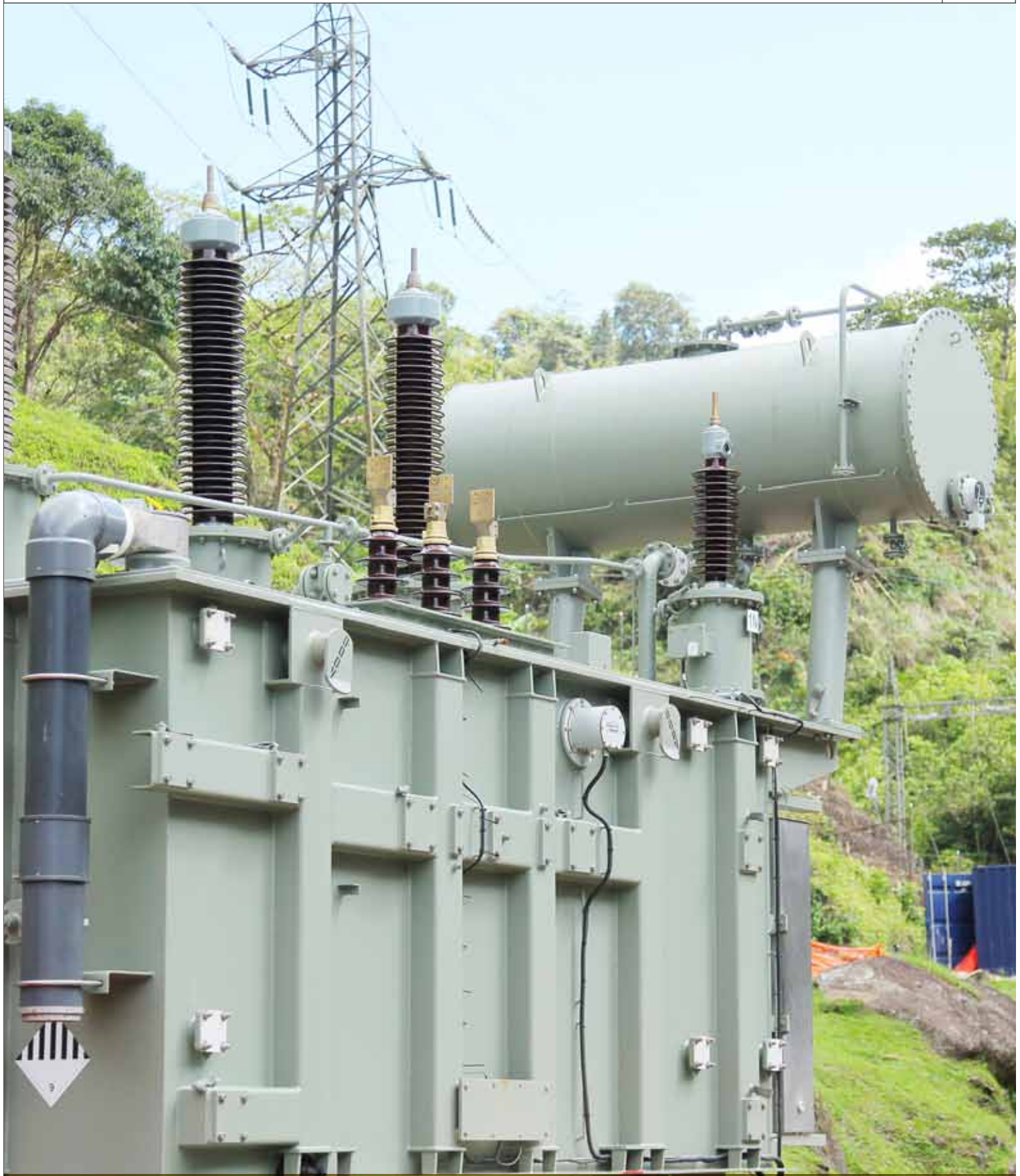
FEA replaced 4x11kV/132kV generator transformers at Wailoa Power Station. These ageing assets have been in service for some thirty plus years. This will improve the reliability and security of power supply to customers in Viti Levu.
